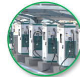
EV Charging Station
